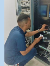
Gosiame Moyo Network Engineer Intern
